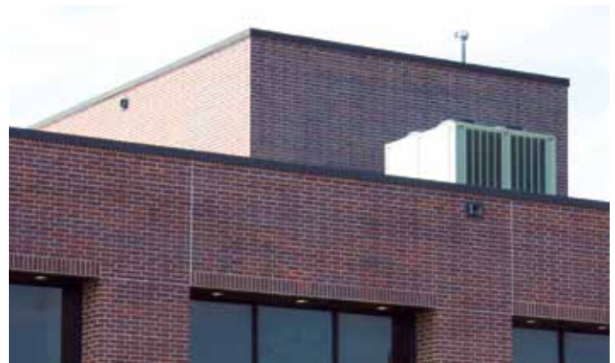
A roof top brick room houses the conventional HVAC equipment.
