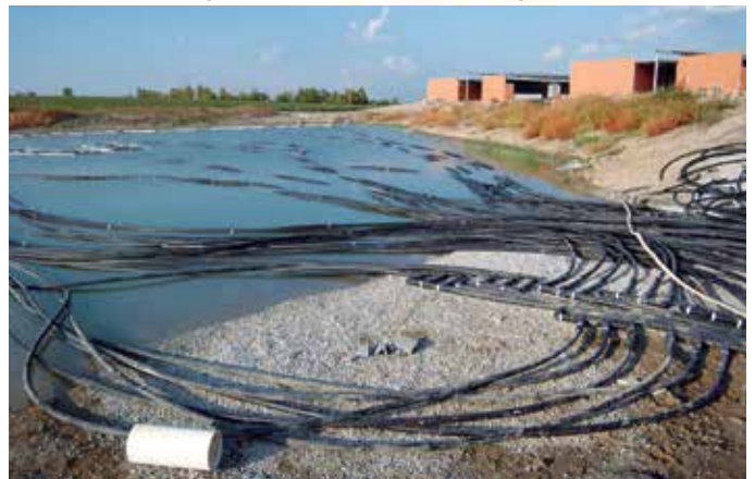
Fused header assemblies for the pond loop system.
