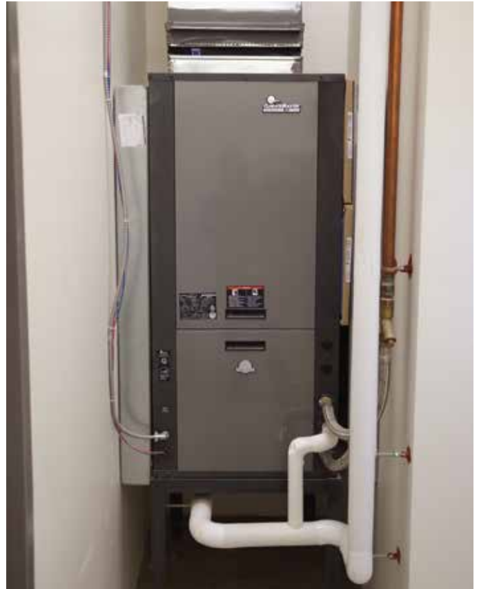
One of the Tranquility 20 Single-Stage (TS) units installed in Falcon Heights
