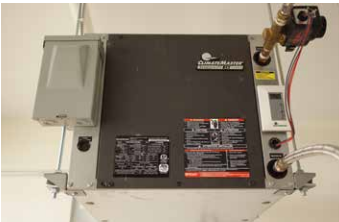
One of the Tranquility® 16 Compact Series horizontal units installed in Centennial Hall
