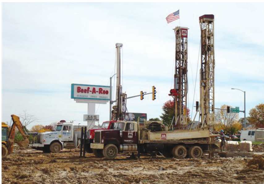
The slab for the 12-shop building was poured in August 2009. The geothermal-exchange field needed to be completed by October, which left just enough time for the parking lot to be paved before asphalt plants closed for the year.
