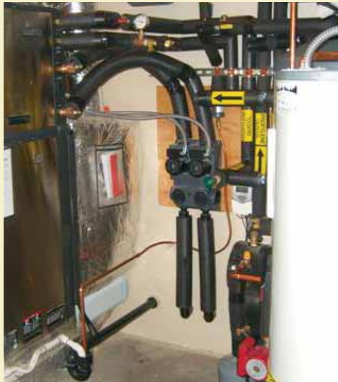
ClimateMaster 5 ton Tranquility 27 geothermal heat pump system.
