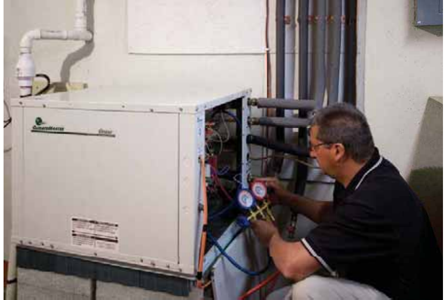
Mark Frost checks the valves on his ClimateMaster unit
