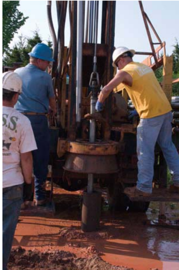
A contractor drills a 400 ft bore to insert a heat exchange ground loop at Hope Crossing
