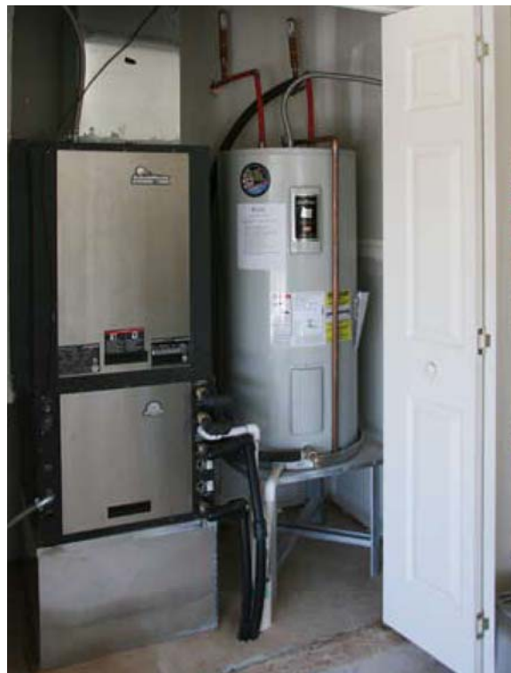
One of the ClimateMaster units installed at Hope Crossing
