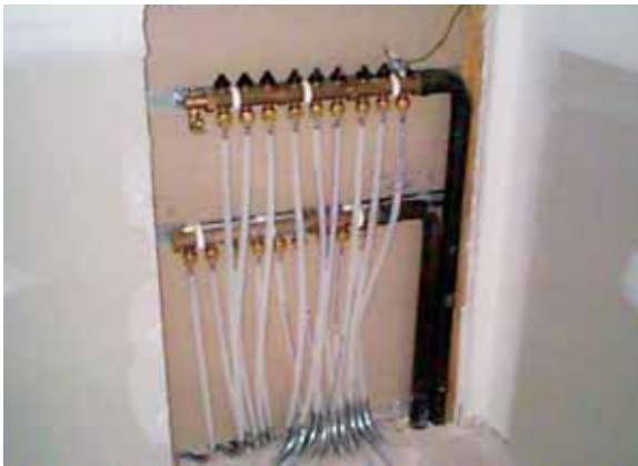
Figure 2-11: Radiant Floor Zone Manifold
